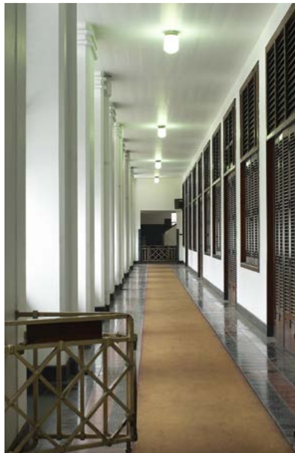
Galleries ensured both natural ventilation and protection from the sun (copyright: ABN AMRO Art & Heritage)
